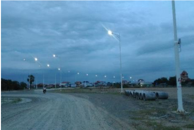
LED street lighting system with wireless network control
