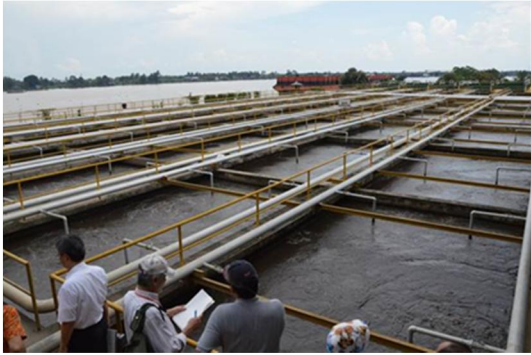
WWTP in PT.ABP
